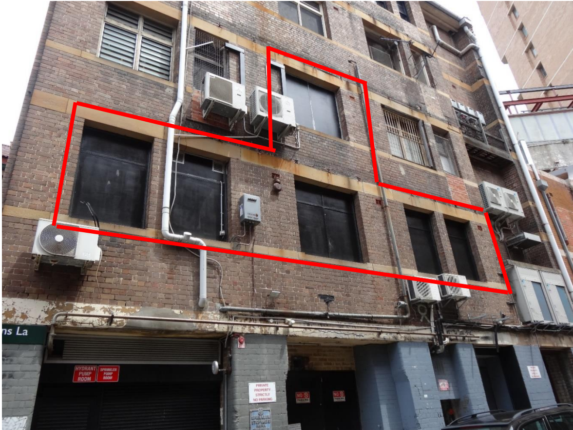
Figure 21: Unauthorised works to the rear windows of the site
